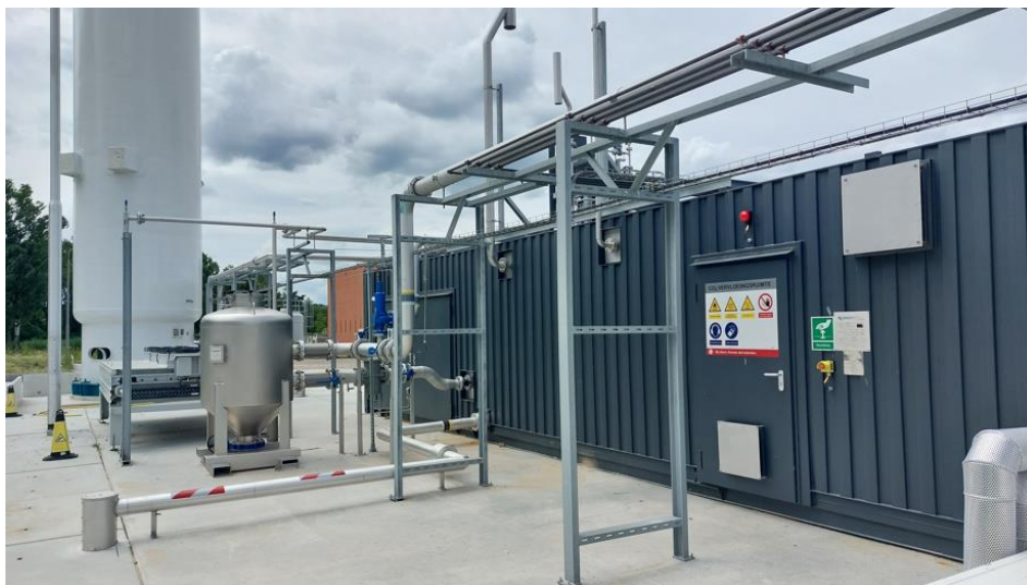
Figure 9 Installation run by the Water Authority The Dommel in Tilburg, where liquid CO 2 and biomethane are produced. (Source: Aquaminerals)
