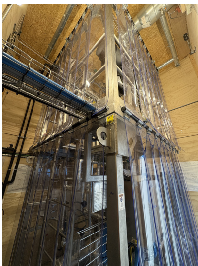
Figure2: DPU1 installation for purification of DME produced in the SEDMES pilot.
