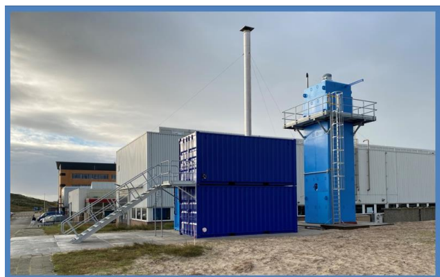
Figure 1: SEDMES pilot facility (3kg/h DME)
