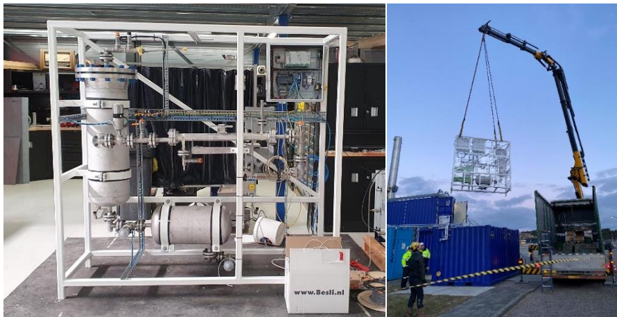
Figure 4: Purge Loop skid. Right: hoisted into the SEDMES container in Petten.
