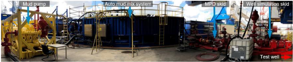
Figure 17: Huisman automated mud mix system to automatically adjust mud properties in real time
