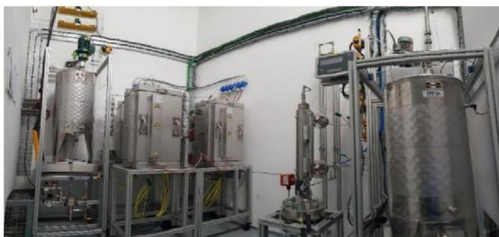
Figure 1: Process Development Unit for the pyrolysis oil hydrotreating
