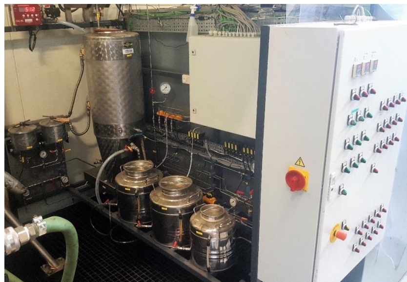
Fig 2: Fuel feeding skid
