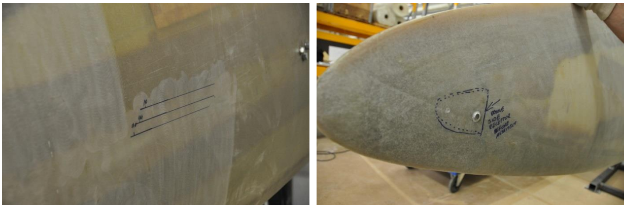
Figure 5-9: Markings on the blade for drain holes and anchor block after grinding
