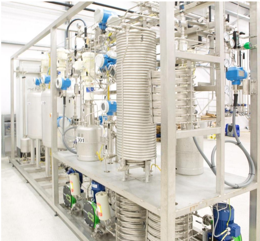
Figure: CADANS skid
