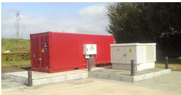
Figure 6: One of the battery storage containers in the pool used for the TenneT FCR pilot
