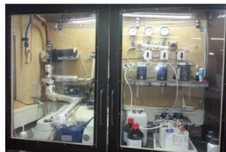
Product gas sampling and conditioning area
