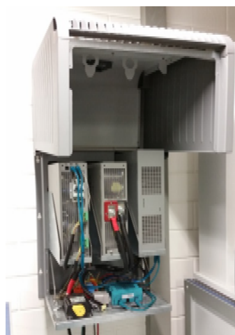
Figuur 8 Storage inverter
